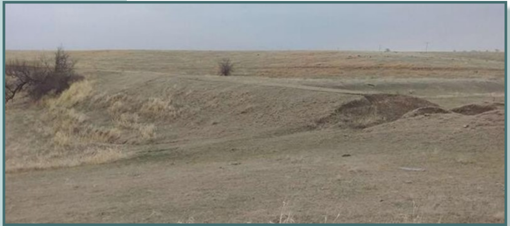
A cattle path cutting through the crest of the dam that was found during the Department's routine inspection can be seen on the right side of the photo. This privately-owned, earthen dam is located less than one mile upstream of Highway 89.
