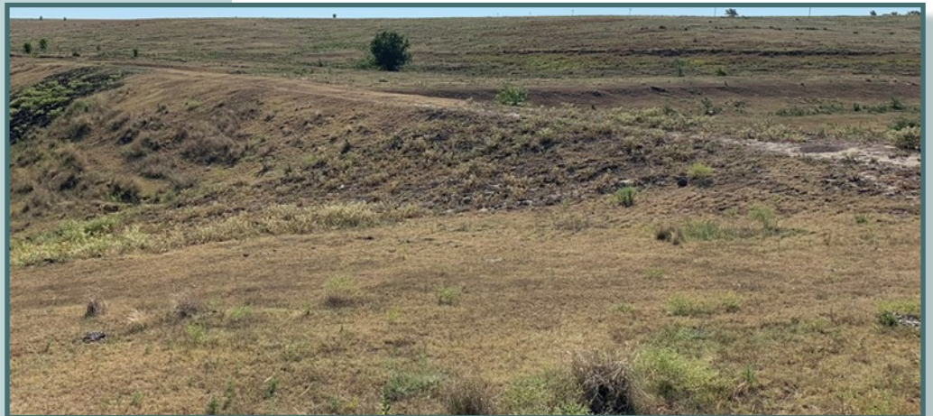
Photo showing the repairs completed by the dam owner after being notified by the Department about the risk the dam posed to Highway 89.
