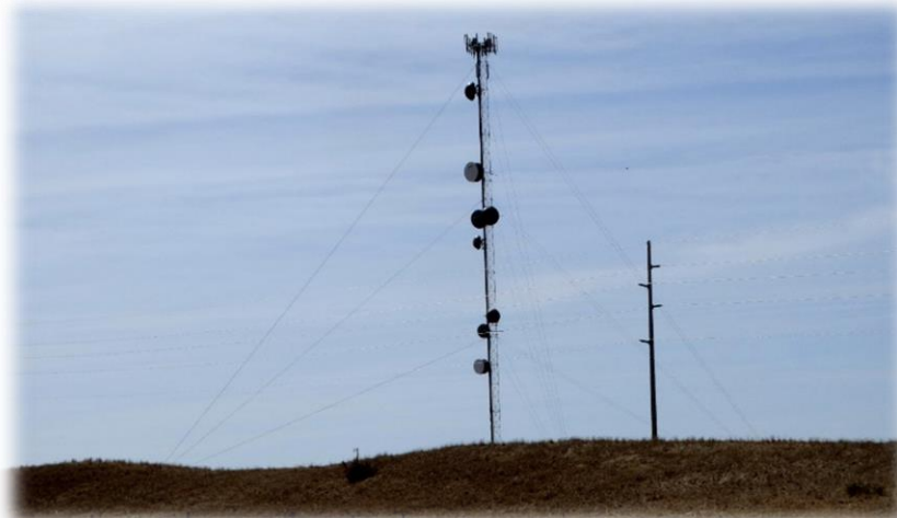
Cell tower-Highway 2-East of Dunning
