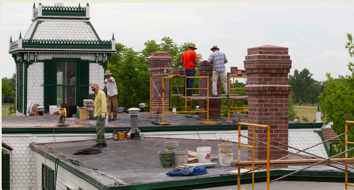
The Buffalo Bill Ranch State Historical Park mansion roof was replaced in fiscal year 2020-21.
