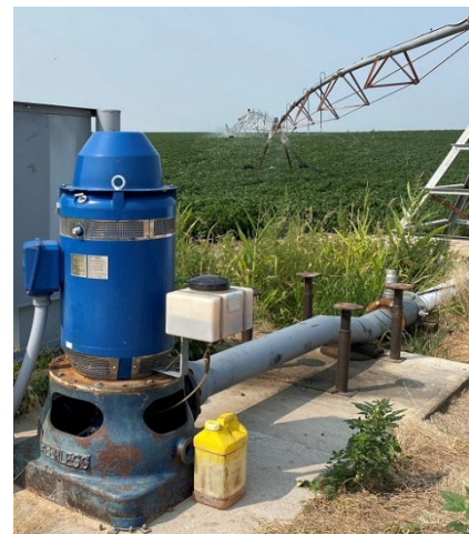
New electric motor at wellsite.
