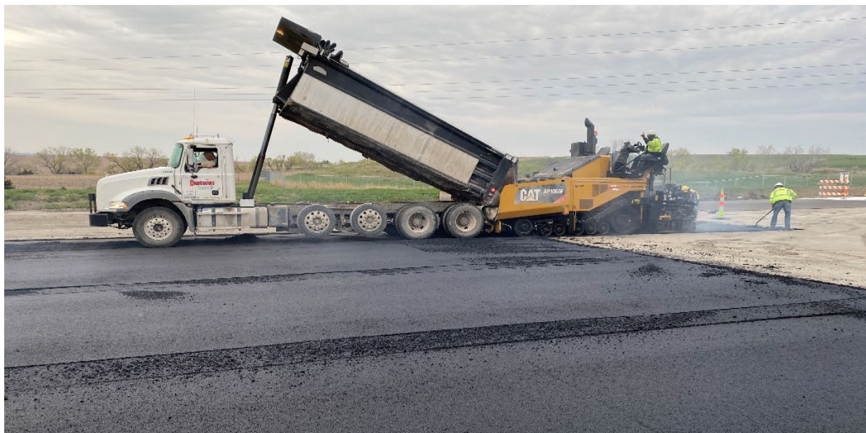
Photo provided by City of Lincoln-Solid Waste Management, which was awarded funding for asphalt pavement repairs for their existing composting pad.
