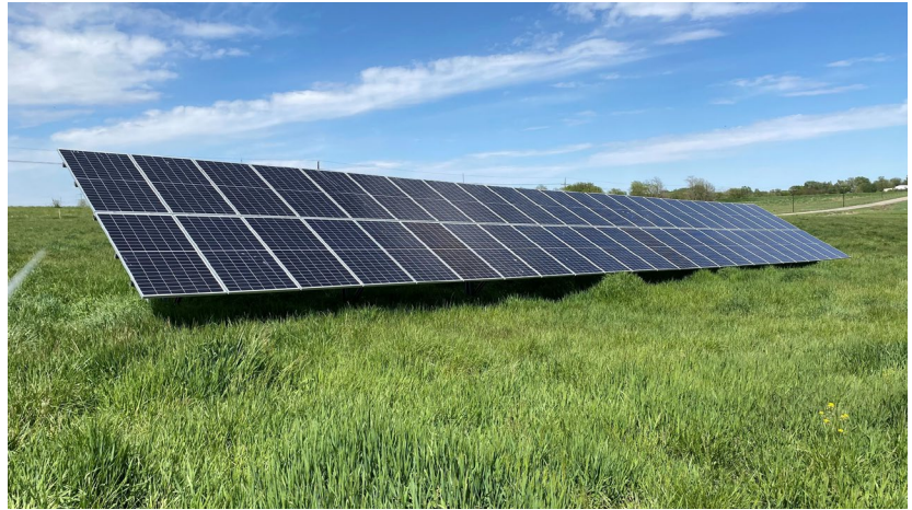
This photo shows a residential solar installation erected summer of 2020 in South Lincoln, funded by a Dollar and Energy Savings Loan from NDEE. Photo by Bryce Puck, May 2021.
