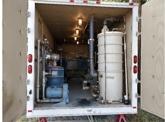
NDEE trailer containing a remediation system
