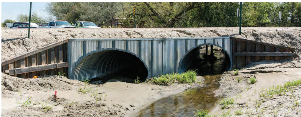
Multiple culvert pipe structures are an inexpensive way to quickly replace structurally deficient bridges.
