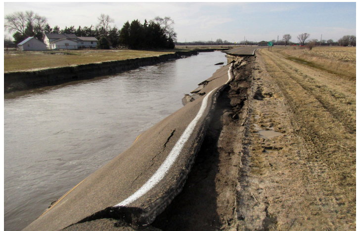
Flooding in March and June 2019 not only damaged roads, it also flooded buildings. NDEE made DESL program funds available at 1% interest to help Nebraskans get back on their feet while making businesses and homes more energy efficient. This picture was taken west of Columbus near Silver Creek.
