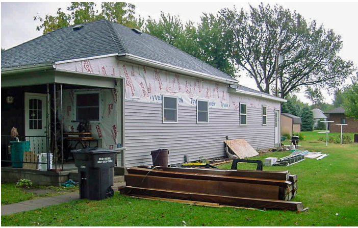
This home in Greeley County received energy efficiency improvements on its doors and windows through the DESL program.
