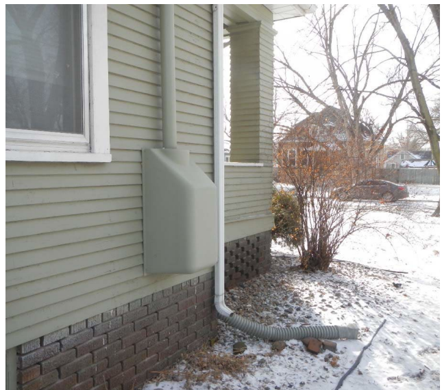
Pictured right: An installed vapor mitigation system at a residence; view is of the installed fan (top) and protective cover (bottom).
