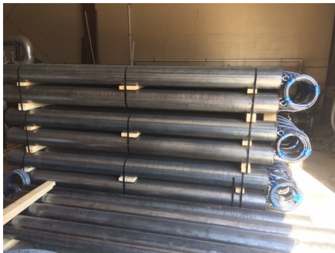
Pictured right: Photos of the in-situ thermal remedy at the Cleburn Street site in Grand Island. During the remedial action, part of the thermal system was installed beneath Eddy Street (top). The installation included electrode wells, temperature wells, extraction wells, and monitoring wells. Heat is generated by the passage of electrical currents between the electrodes (bottom).
