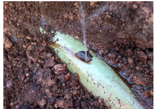
Active leak in Chadron
