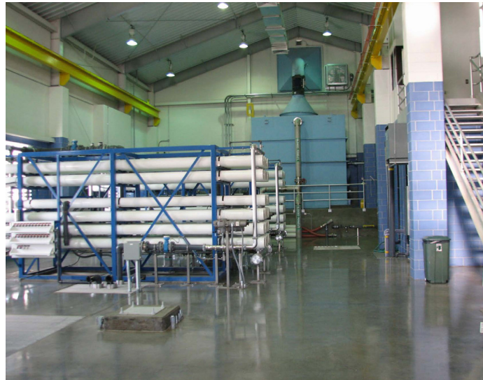
Reverse Osmosis treatment plant to remove nitrate (Seward, NE).
