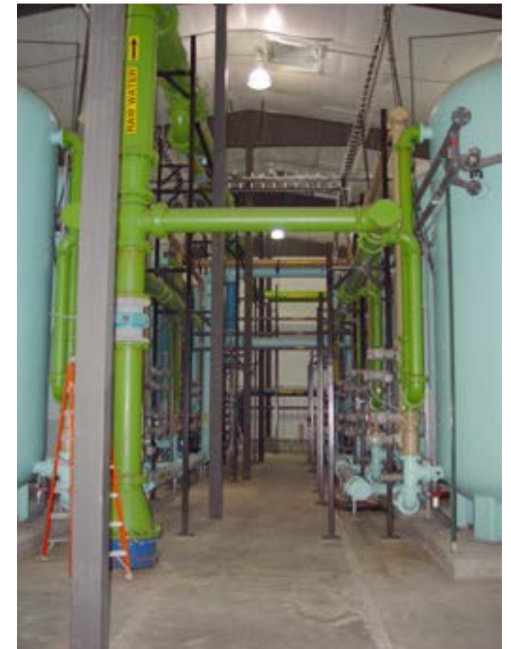
Ion Exchange plant to remove uranium (McCook, NE).
