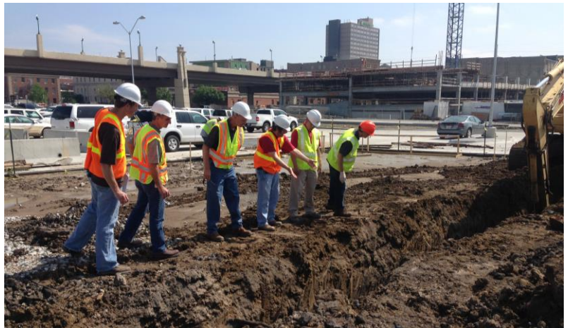
Staff of NDEQ, the City of Lincoln and its contractor observe remediation at the West Haymarket Voluntary Cleanup Program site in Lincoln. See page 35 for more information on the Voluntary Cleanup Program.
