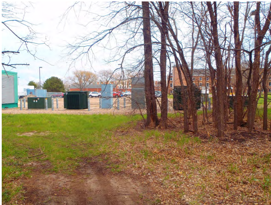
Photo 17: Utility equipment (electrical and otherwise) for the existing Veteran's Home located east of the assessment property. Electrical equipment did not have "No PCB" placards.
