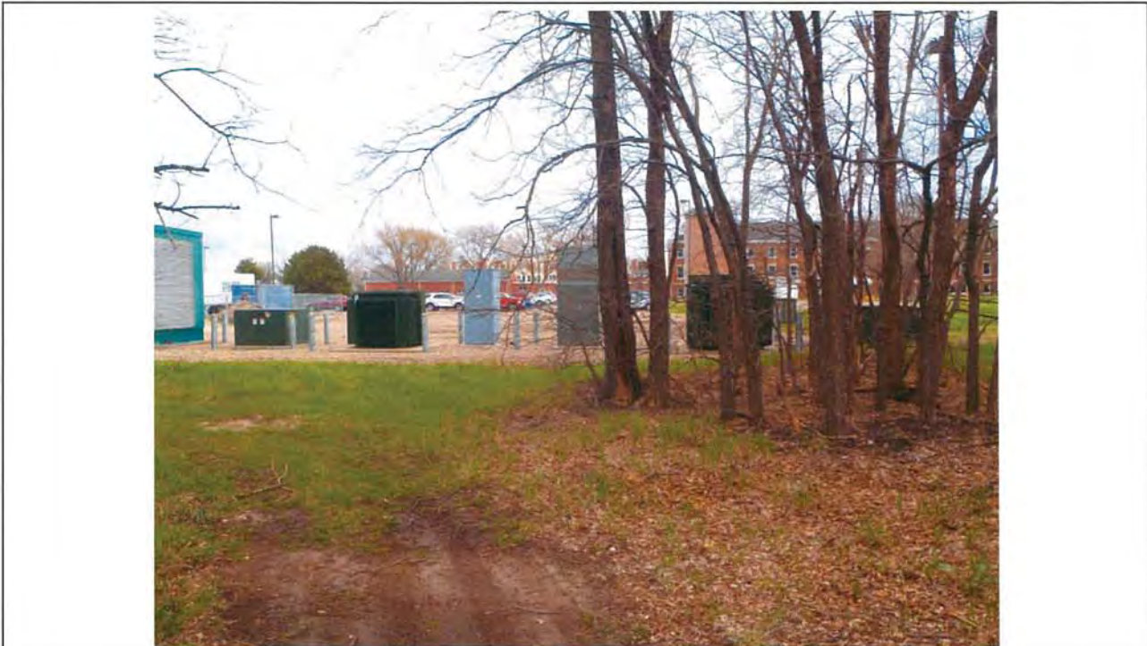
Photo 17: Utility equipment (electrical and otherwise) for the existing Veteran's Home located east of the assessment property. Electrical equipment did not have "No PCB" placards.
