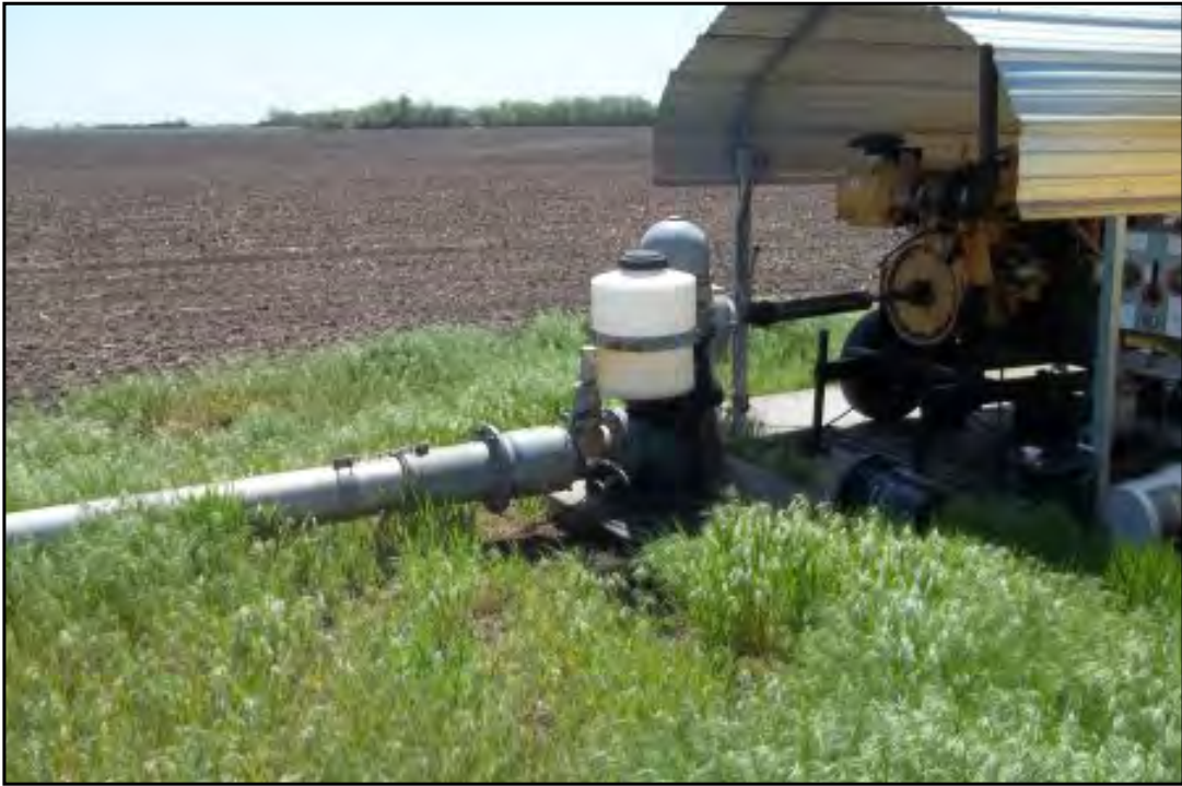
Irrigation well with some soil staining.
