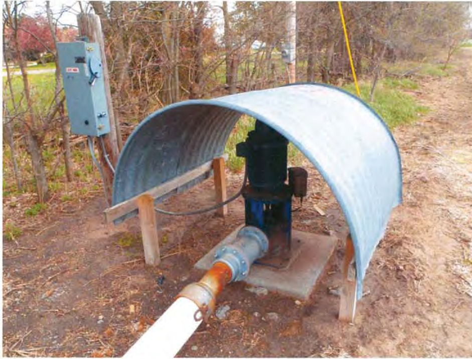
Photo 5: One of two irrigation wells located on the assessment property. This well is located along the southern boundary of the property. The irrigation well was electrically powered.
