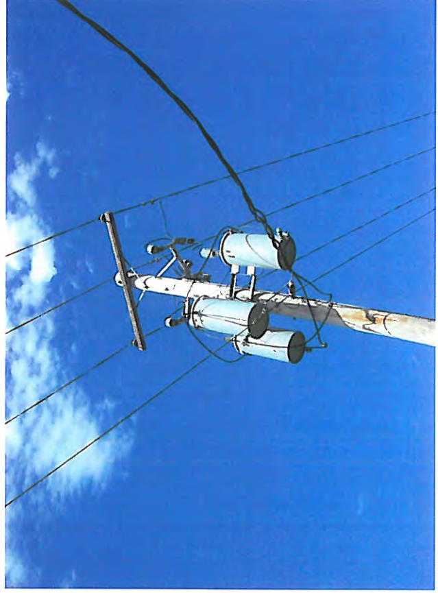
Photo 16: Three Transformers on Pole, Northeast Corner
