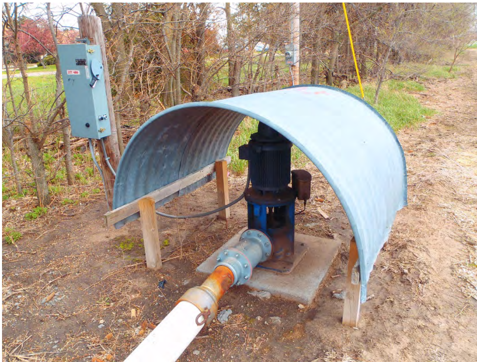
Photo 5: One of two irrigation wells located on the assessment property. This well is located along the southern boundary of the property. The irrigation well was electrically powered.
