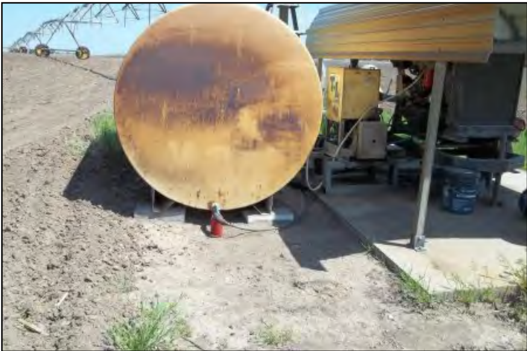
AST, motor and oil for irrigation well
