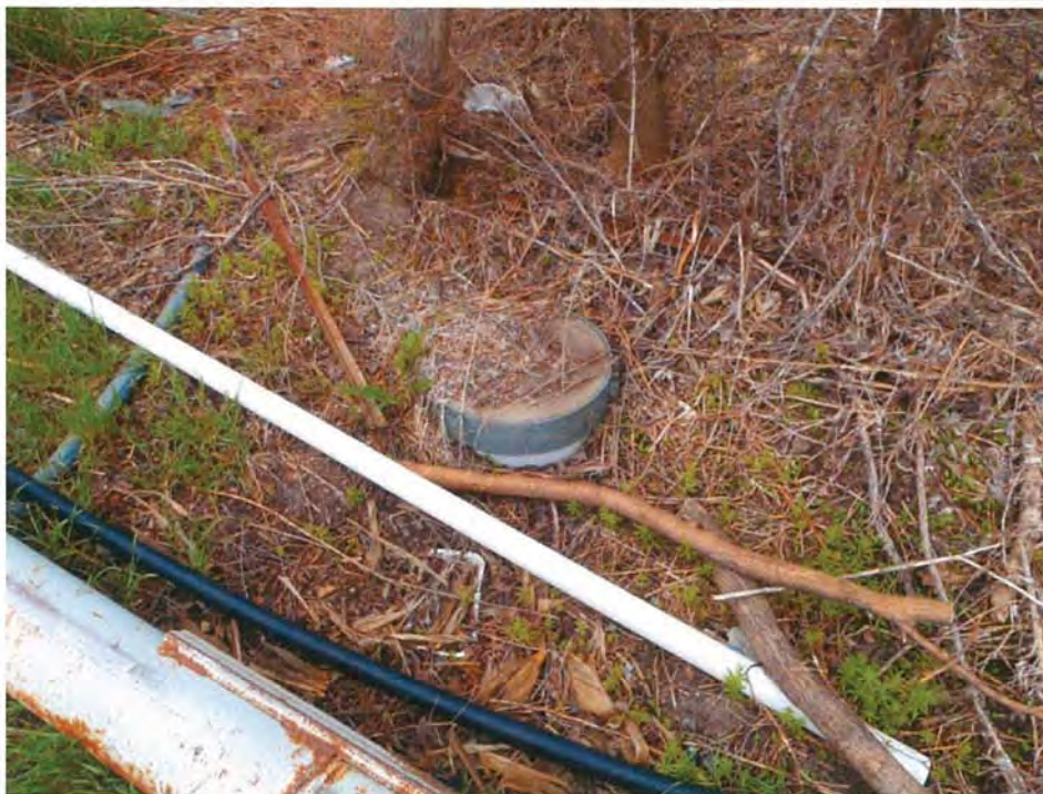
Photo10: Small manhole noted near the irrigation well in Photo 9. The function of the manhole was not evident.
