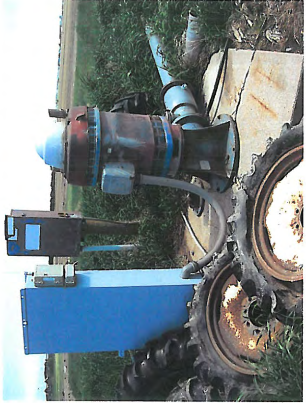
Photo 15: Irrigation well-Northeast Corner.
