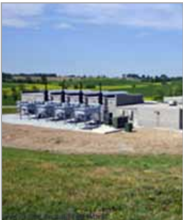
OPPD's Landfill Gas Plant near Elk City
