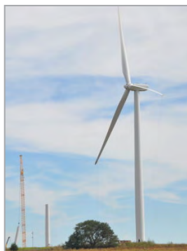
One of 44 turbines for the Steele Flats Wind Project rises from the ground near Diller.
